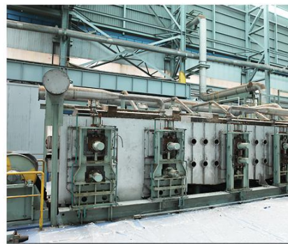
step2 PRE CLEANING To eliminate foreign substances from the strip surface, hot alkali solution is sprayed onto the strip surface.
