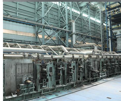
step4 CLEANING SECTION Consists of 5 steps: clearing, brushing, rinsing, hot water rinsing, and final rinsing. While removing foreign substances from the strip, a chemical agent is applied to improve adhesive strength. Processing time of 7-9 seconds and length of 16 meters. (LS 120 MPM)
